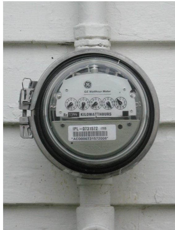
Figure 2 – typical 60A S-Base meter
